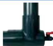
Installation of valves and cocks for sampling and draining.
